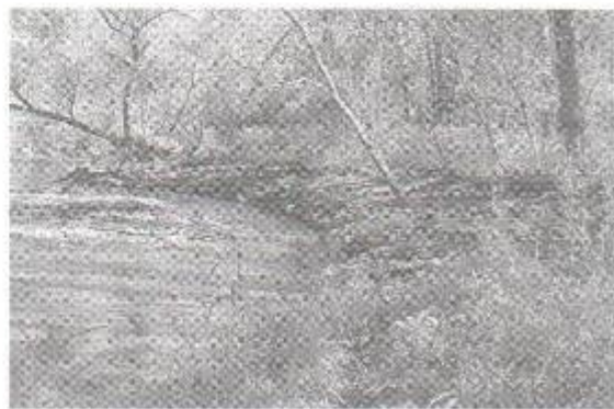
Finished stream bank. Lumber structures buried at edge of stream bank provide cavities for fish to hide in. Trees over stream have been left for habitat, benefitting birds and fish.
