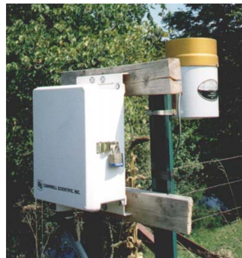
Figure 1 Datalogger and rain gauge
